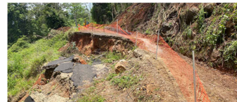
Tuntable Creek Road post-landslip in 2022.
