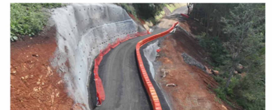
The temporary fix in 2023.
